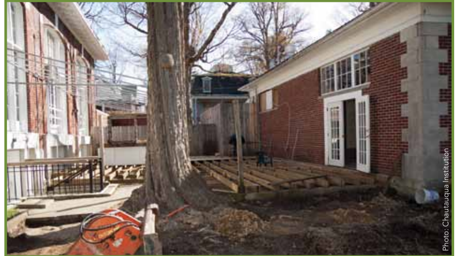
Current progress on spring construction of the deck between the Refectory and the Post Office building.
